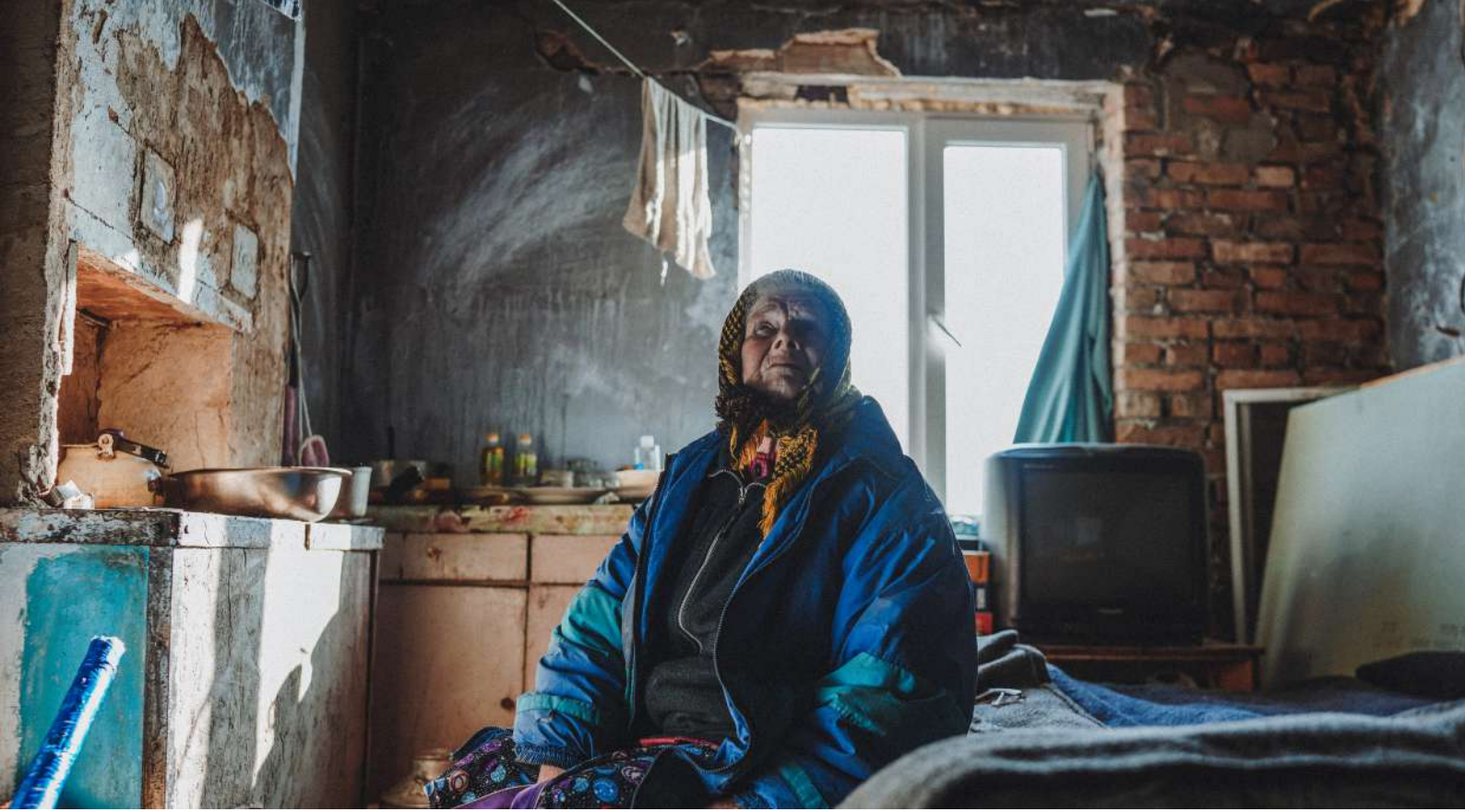
Figure 13 The blackened walls and ceiling are a daily reminder for Rosali (82) of the fire that broke out when her house got shelled. She spent some nights in one corner of the house that was still a bit dry, because rain kept pouring through the holes in her home.
